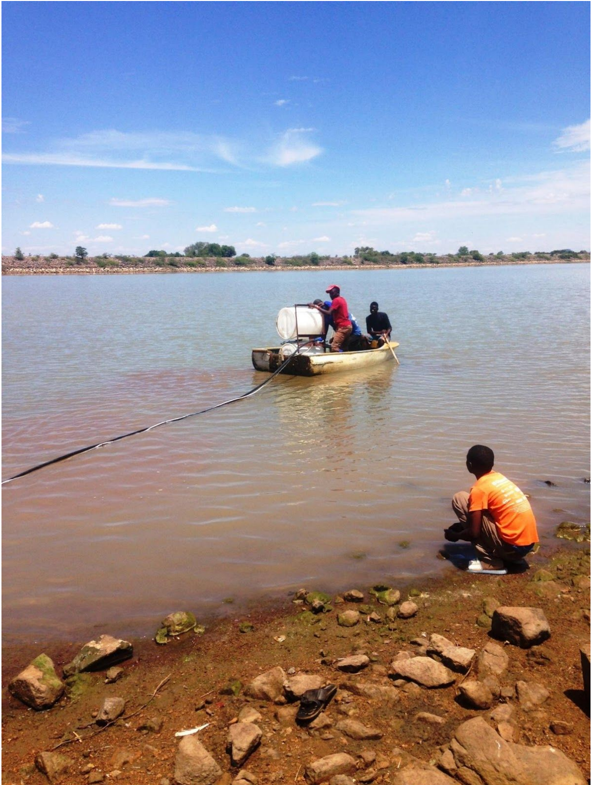
The engineers had to extend the length of the conduit beyond 250m to place the pump deeper inside the dam.
