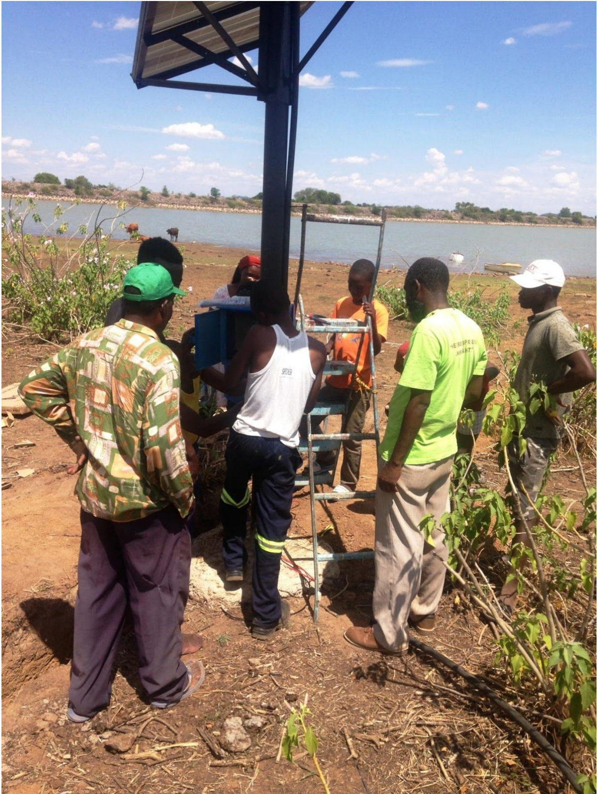
The solar source of power for the water pump
