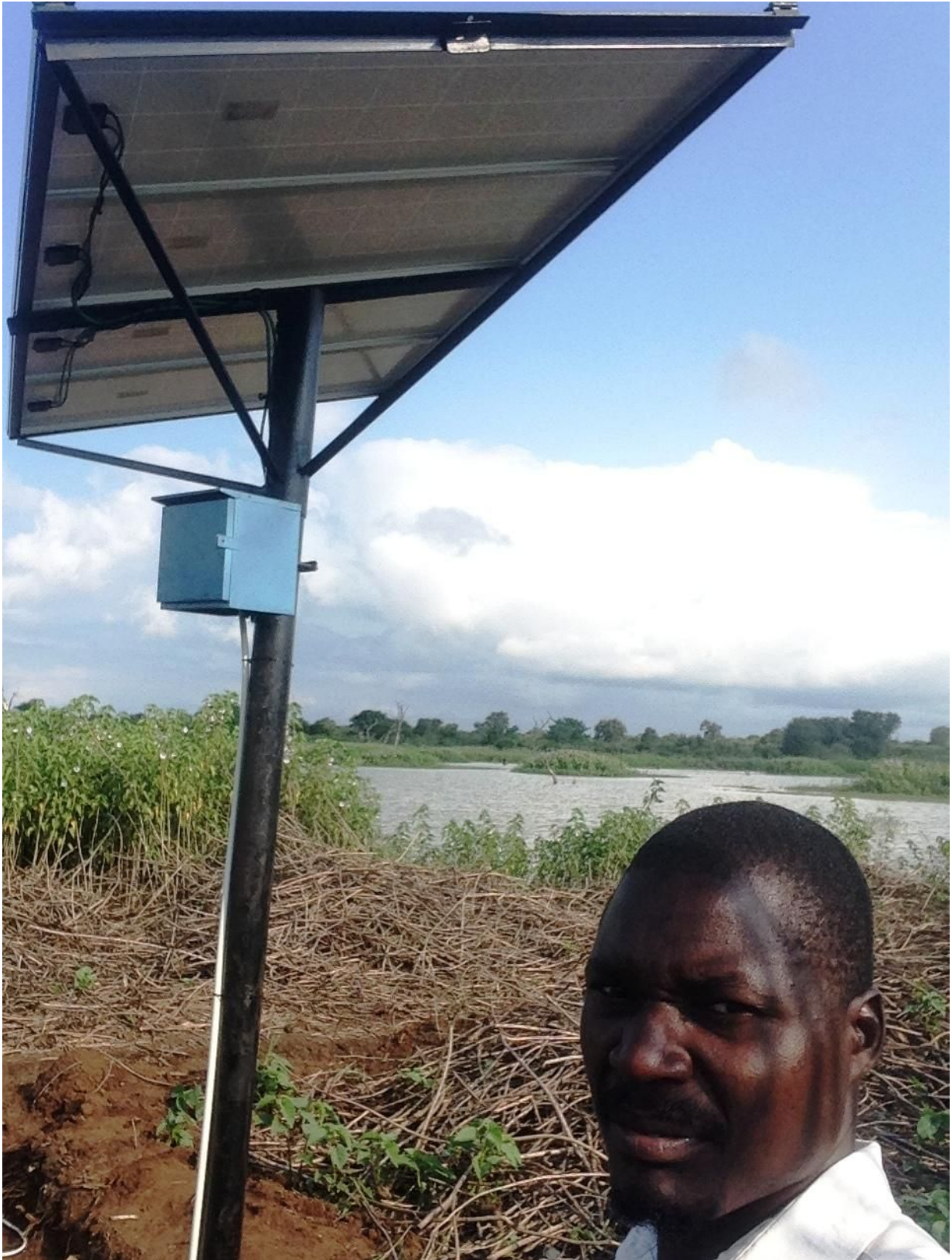
The power source for the submersed pump
