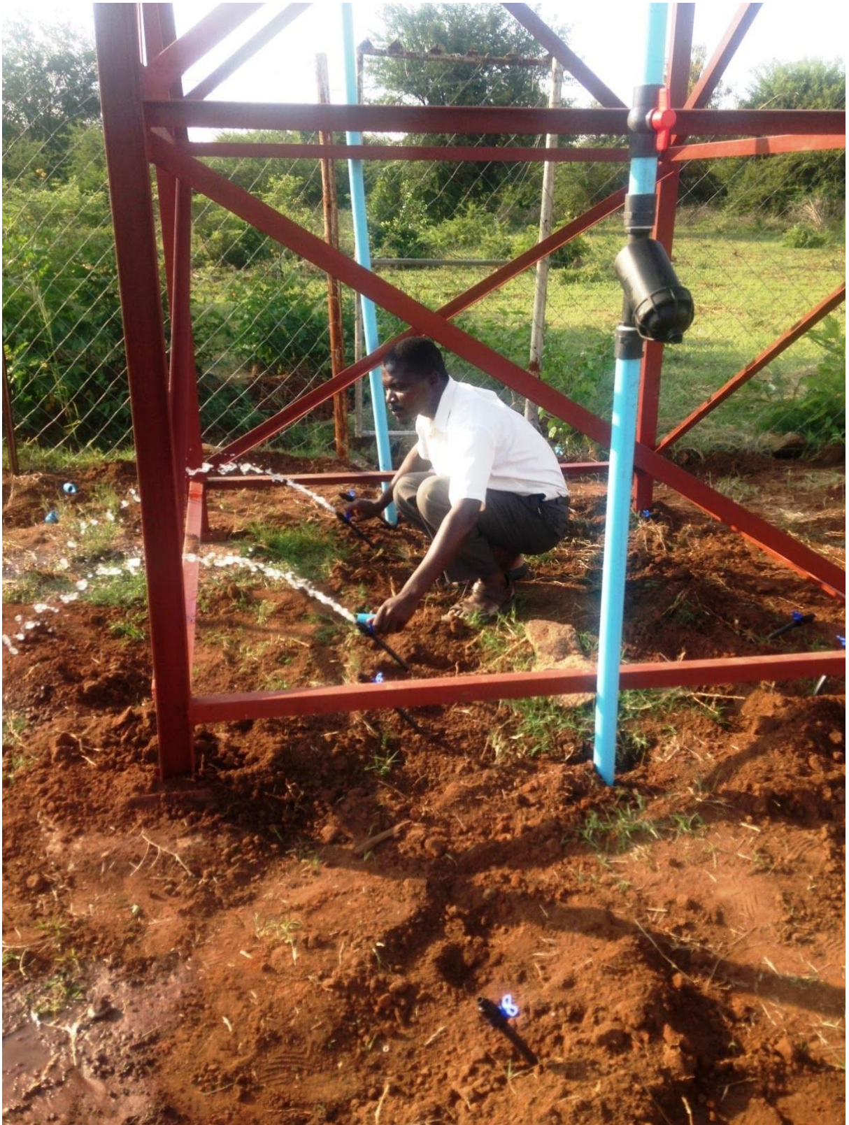
Testing the pressure of the pumped water on a rather cloudy day, before the tank was even filled
