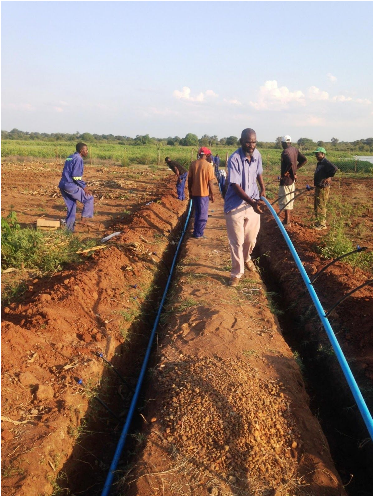
The Agric Officer (in the foreground and facing the camera) participating in laying the pipes
